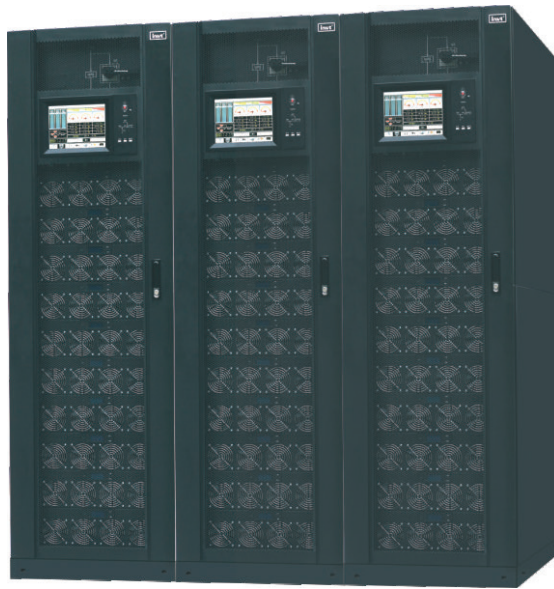
Three units in parallel
